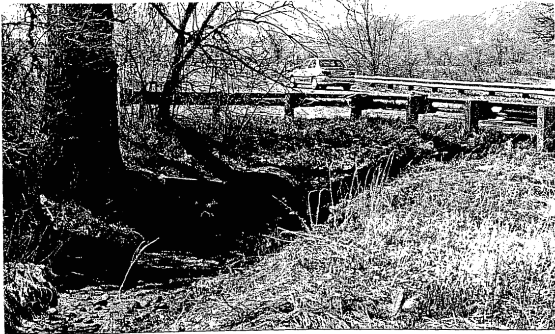
Photo 3. This is the east side of East Boulder Ditch (Work Zone 3); the culvert will be extended but with work conducted from the road. 4/18/01
