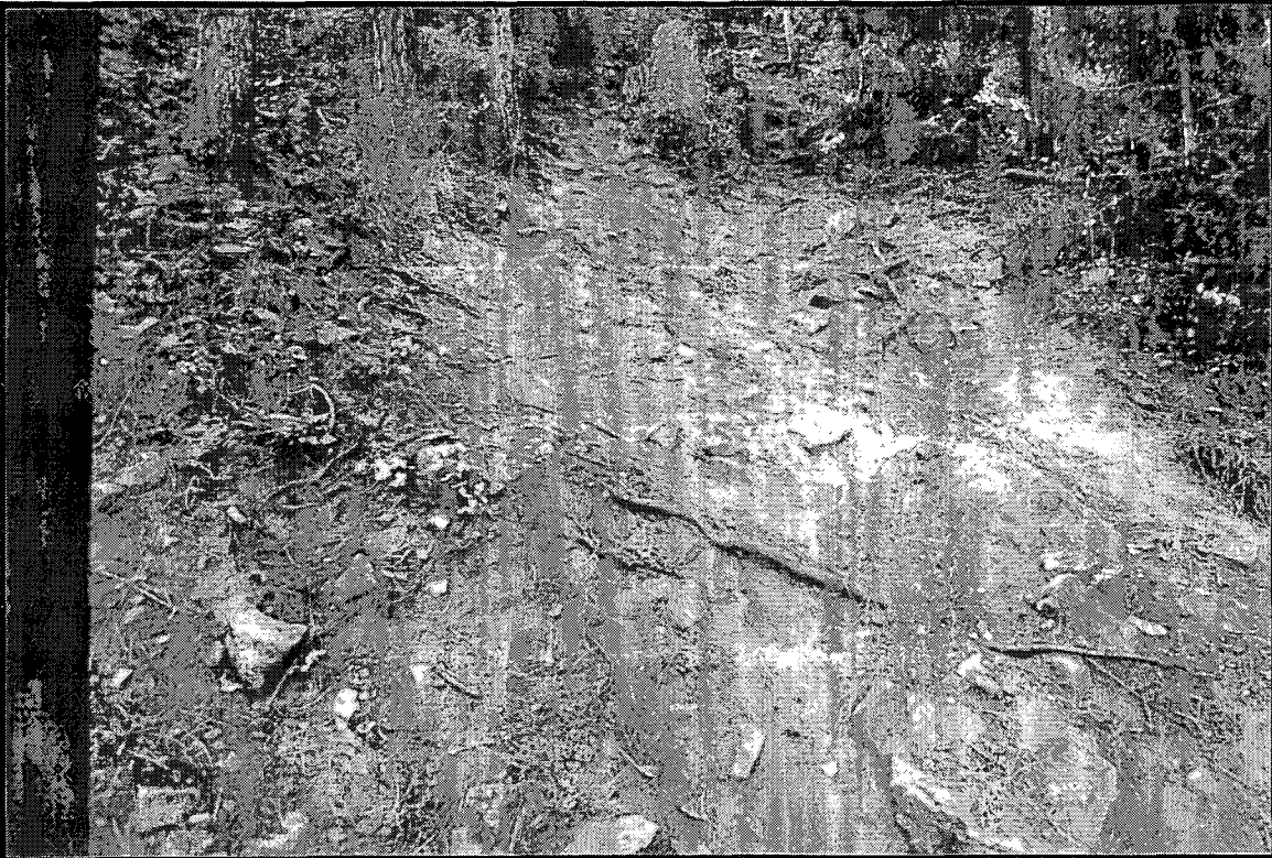
PHOTO #1: Erosion between Gregory Canyon and the Amphitheater, looking south.
